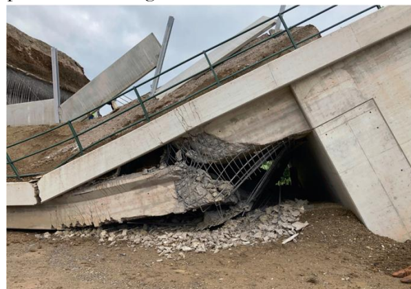
Figure 2. Shear failure of Wieselburg bridge [6]
