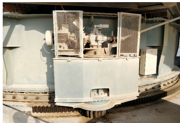
Figure 11. Electrical motor, swing drive, manual operation crank, pinion and gear at pier.
