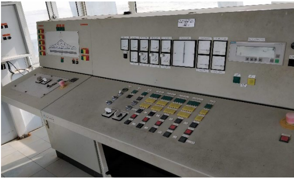
Figure 13. Bridge panel control in the EB
