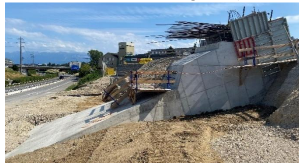
Figure 18. Partially buried abutment
