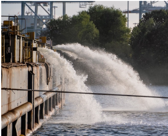
Figure 2: Detail of 3 of the 12 900 m 3 /hour pumps
