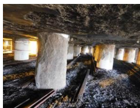
Figure 8. Columns. Spalling shallower than 25 mm
