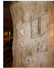
Figure 5. Columns. Concrete cover spalled, long rebars exposed
