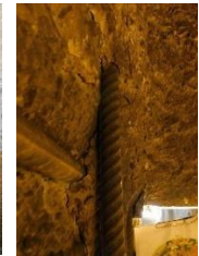
Figure 7. Splitting. Loss of bond between concrete and rebar
