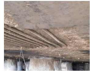
Figure 4. Slab. Concrete cover spalled, 1 rebar layer exposed
