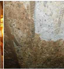
Figure 6. Progressive spalling. Notice the different concrete colours
