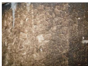
Figure 9. No spalling but cracks visible on the surface
