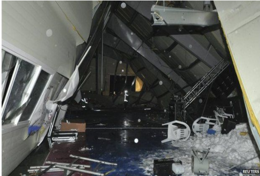
Figure 3: Collapsed frame-type roof structure with life-saving spaces inside the building [25]
