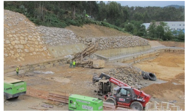
Figure 9. Execution of the top row of ground anchors with temporary pile wall protection and backfilling of the excavation.
