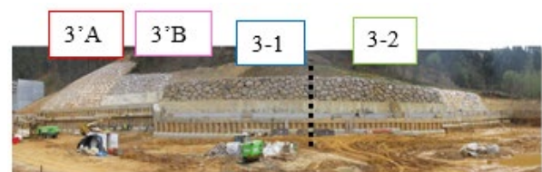
Figure 1. General view of the pile wall. Critical zone in April 2014, before reaching the maximum level of excavation.
