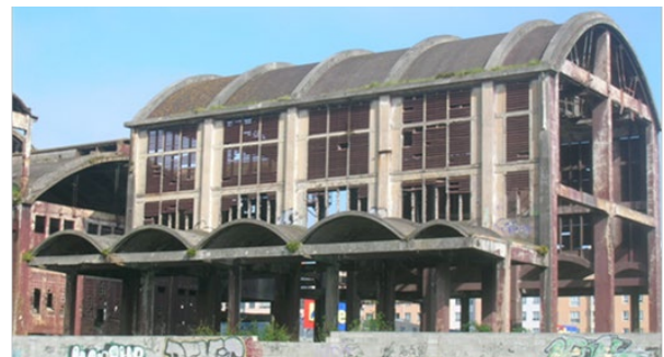
Figure 1. Condition of the industrial building before transformation (Courtesy of Diaz & Diaz Architects S.L.).
