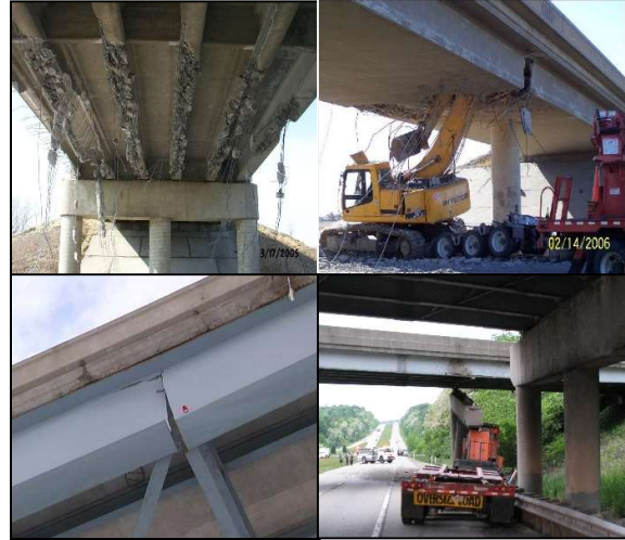
Figure 1. From top left clockwise – all girders damaged in multi-girder concrete bridge, superstructure cut-through in concrete box girder bridge, pier damage and support loss in multi-girder steel bridge, and through girder fractures in a three-girder bridge where all three girders were damaged.
